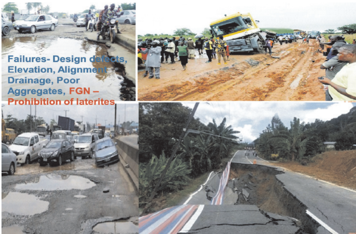
Fig.12: Pavement conditions in sections of the Niger Delta.
