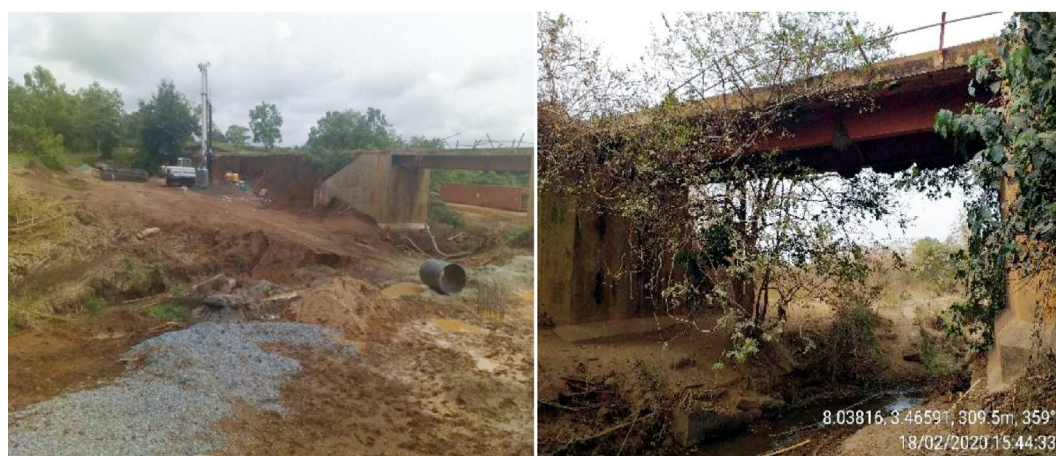
Fig. 3: Skewed and dilapidated existing Okeho bridge
