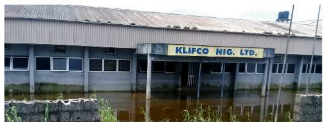
PLATE 4: Flooded Klifco company in August 2017
