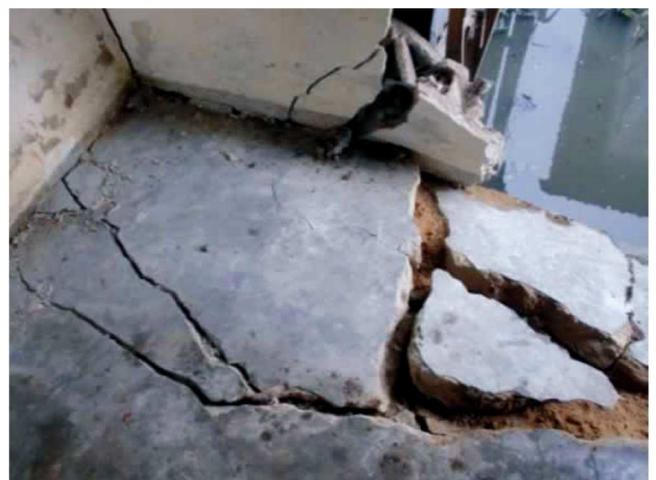
Collapsed building after earthquake at Igbogene, Bayelsa. Photos: Tobi Aworinde and CGG
