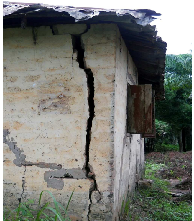
Fig. 1: Evidence of failure of engineering structure due to swelling in Enuguss Shale
