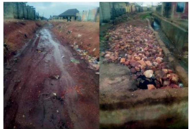
Plate 9: (left) wash away access road by erosion at Barkin Sale area (9° 35'8"N, 6° 31' 29" E)
