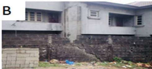
B House experiencing partial settlement at Medina Estate, Lagos State.
