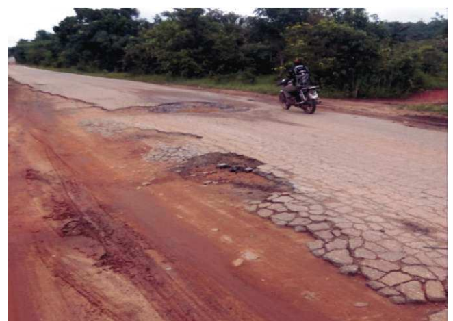
Fig. 3: Plate Showing distressed portion of Station C3 along Igarra- Ibillo Road.
