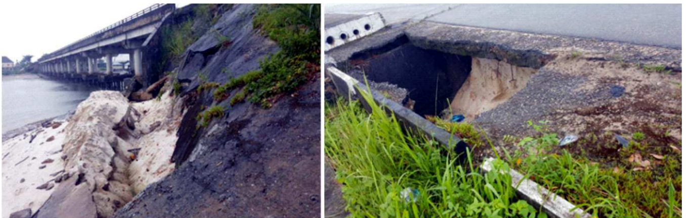
Fig. 6: Erosion of Abutment base and failure of asphaltic surface
