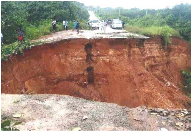
Fig. 6(b): Erosion site between Abia State University and Nkwonta along Uturu - Isuikwato Road, 2018
