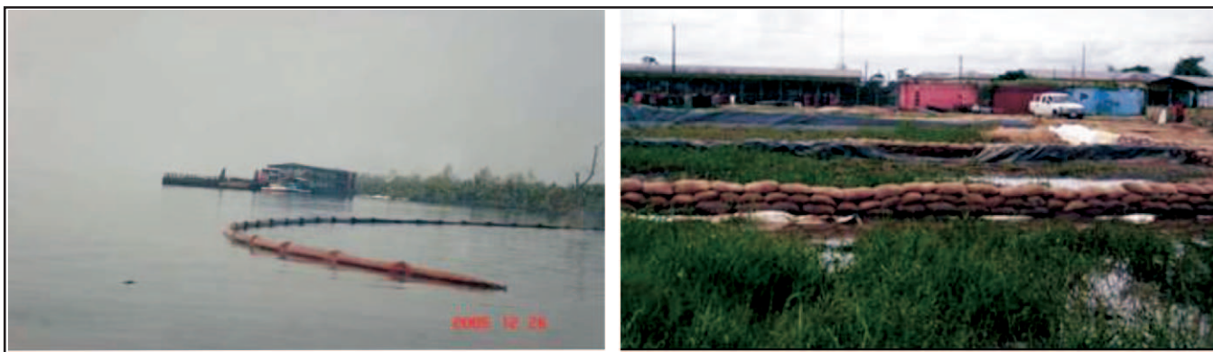
Fig. 3: Oil Spill Containment by River Boom Deployment on Water and Sand-bag Dike Used to Contain Spilled Oil on Land
