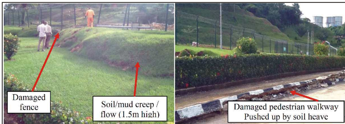
Fig. 7(e): Photographs showing soil plastic/liquid flow and creep causing severe damage to concrete drains, concrete roadside pedestrian walkway and fence
