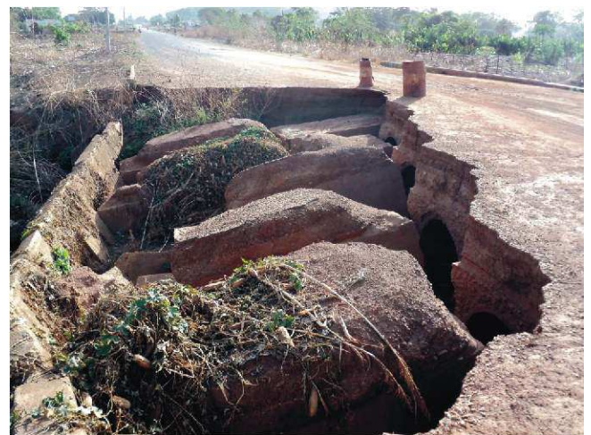
Fig. 8: Typical pavement failure due to poor quality soil
