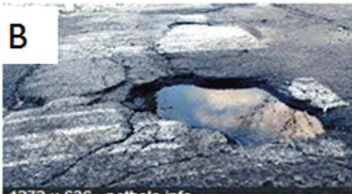
B Small potholes, showing isolated failures of the pavement and its subsurface structure Ref: https://en.wikipedia.org/wiki/Pothole
