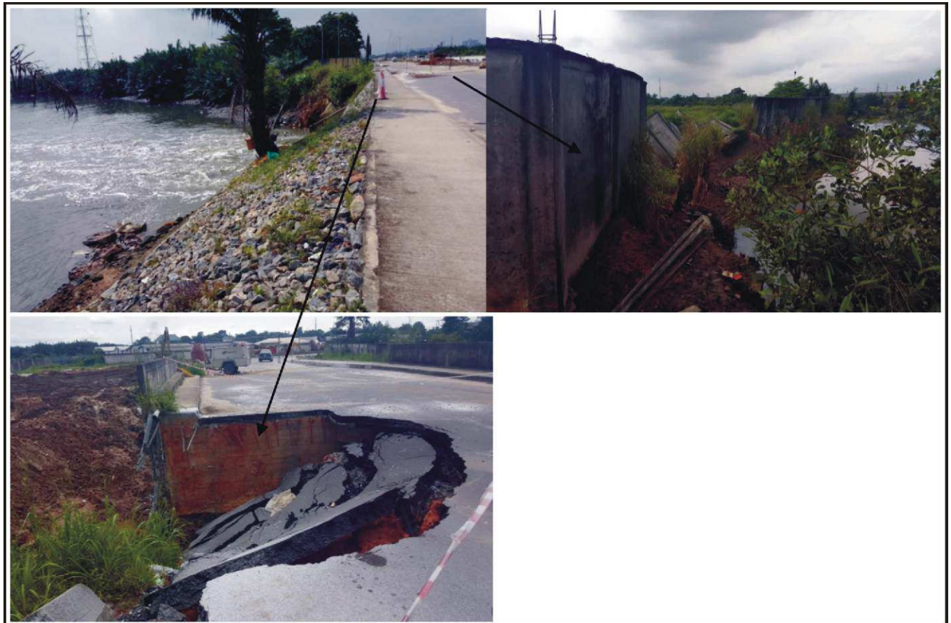
Fig. 7: Failures due to erosion of bridge abutment at Nkpogu
