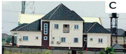
C House experiencing partial settlement at Ash, Lagos State.
